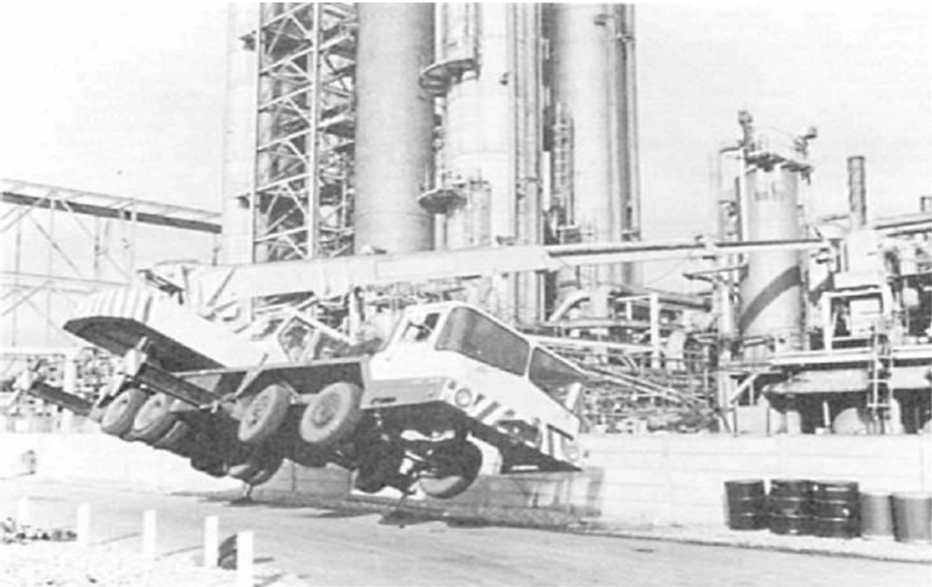
Mobile crane overturned on to plant (Anon., 1977n)
